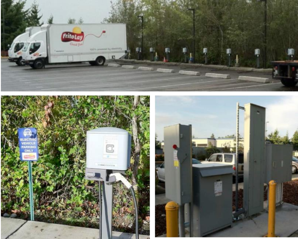
Figure 48. Ten Charging Stations and Facility Power Supply (NREL) [89]
