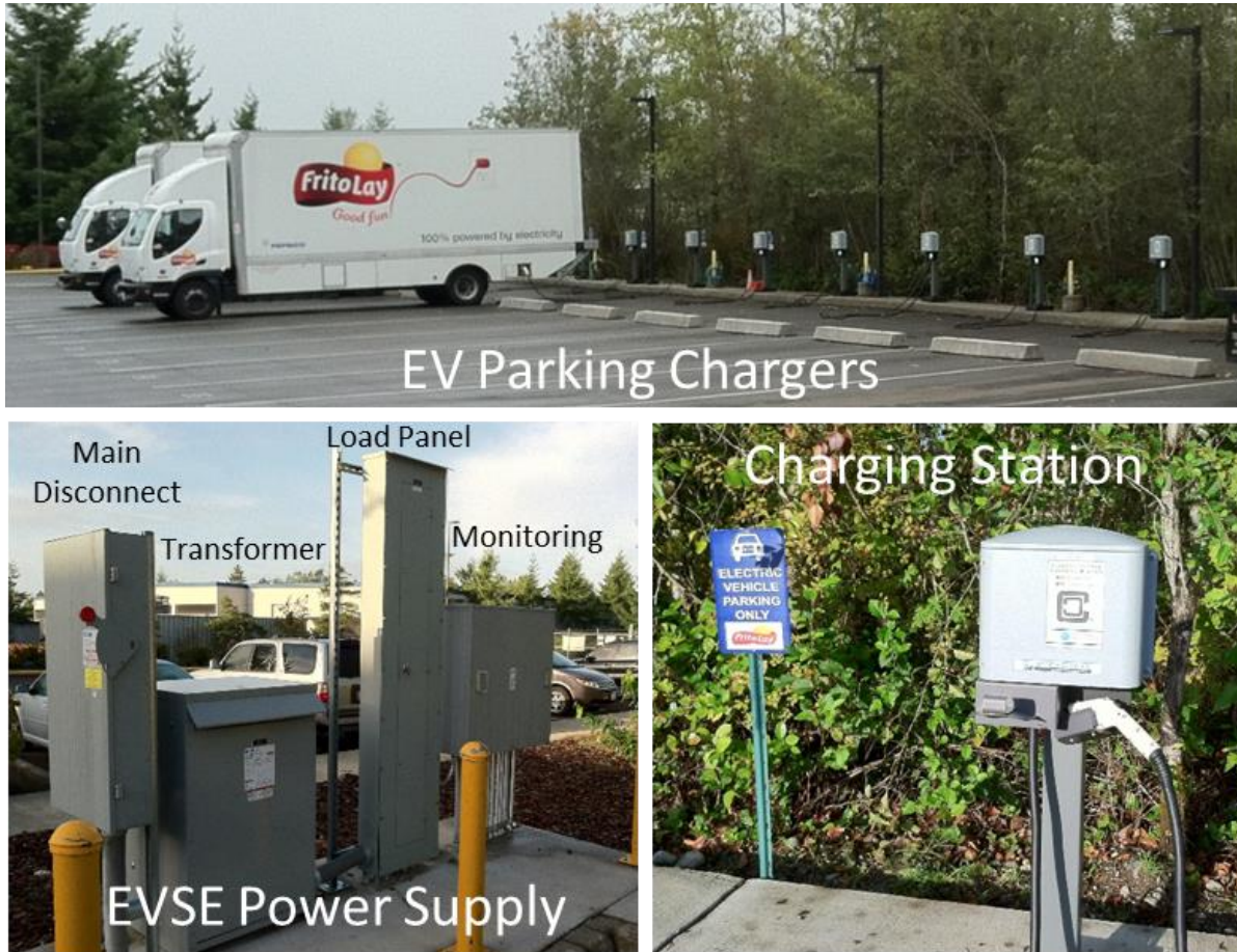
Figure 9. Ten Charging Stations and Facility Power Supply (NREL) [12]
